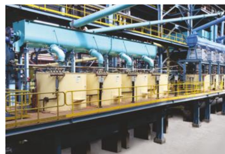
Common Steam Distribution Header
